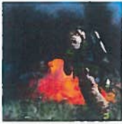
A firefighter closely monitors the fire demolition of the old Fallbrook Golf Club, March, 31.
