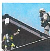
Various San Diego County firefighters train and utilize as much of the old Fallbrook Golf Club structure as possible to learn about structure fires and fire behavior. The “real world” site is ideal for learning, compared to reusable fire facilities that firefighters tend to memorize.
