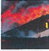
The old Fallbrook Golf Club structure becomes fully engulfed in flames during a demolition conducted by firefighters from throughout northern San Diego County.
