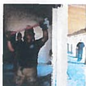
Rincon firefighter Marco Gonzalez uses a sledgehammer to punch holes in the walls of the old Fallbrook Golf Club structure before a big burn demolition of the building, March, 31.
