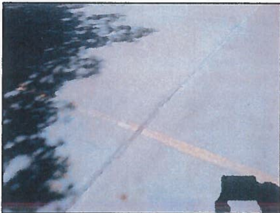
Photo 3 Maintenance Facility – Concrete driveway expansion joint seal failure and faded striping
