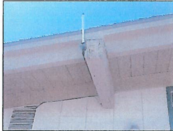
Photo 2 Fire Station 2 - Mild weather at end of exposed beam
