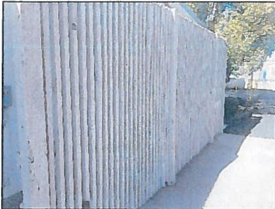
Photo 5 Fire Station 1 – Shade wall showing deterioration
