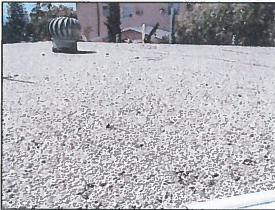
Photo 7 Communications Annex – Roofing material is aged and in poor condition with advanced degradation at perimeters.
