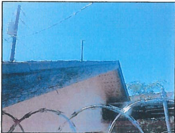
Photo 3 Communications Annex – Aged fascia boards
