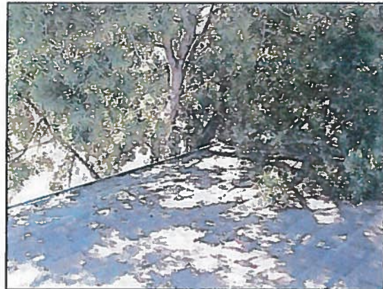
Photo 6 Fire Station 6 – Tree overgrowth onto roof
