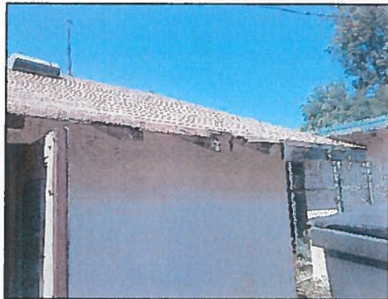
Photo 2 Communications Annex – Visible deterioration along roof decking edge where fascia board is missing
