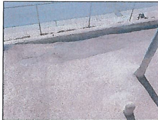
Photo 10 Fire Station 1 – Signs of poor roof drainage
