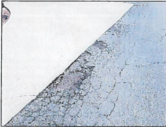
Photo 1 Fire Station 3 – Cracks in concrete driveway and severe cracking and spalling of street asphalt along driveway
