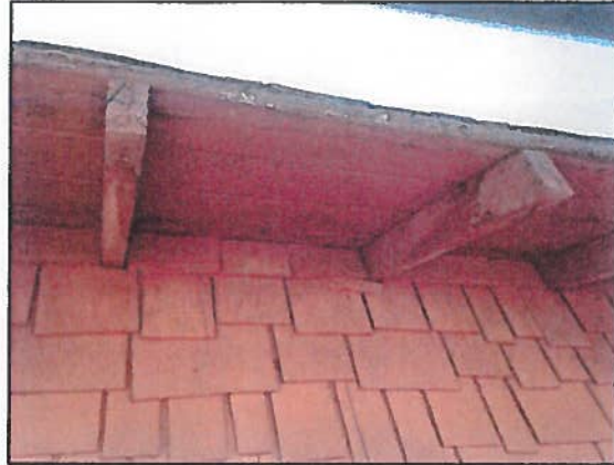
Photo 6 Roy Noon Meeting Hall – Rot and deterioration along edge of roof decking and visible weathering in rafter tails
