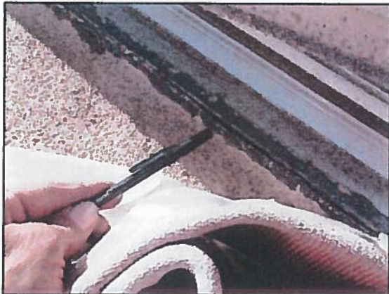
Photo 11 Fire Station 1 – Failed seal around skylight
