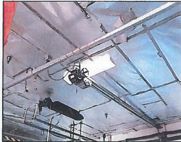
Photo 10 Fire Station 6 – Belt/chain operators service neglected
