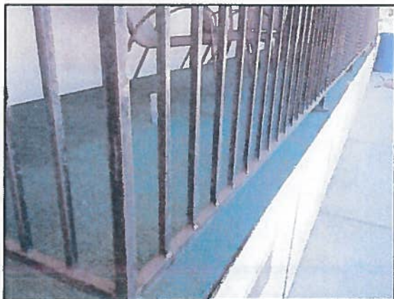
Photo 4 Fire Station 4 – Front ramp railing paint is failing and outdoor carpeting is highly worn
