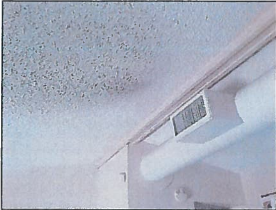
Photo 17 Fire Station 4 – Stains around vent suggest inadequate air filtration
