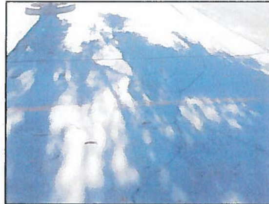
Photo 2 Fire Station 6 – Cracks in concrete parking area
