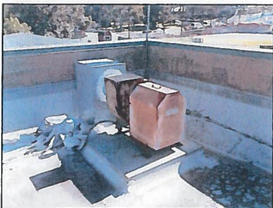
Photo 13 Maintenance Facility – Exhaust fan exterior exhibiting surface rust
