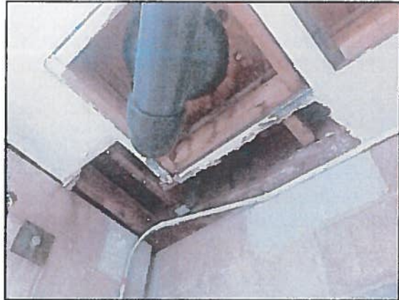
Photo 10 Maintenance Facility – Ceiling damage due to previous roof leak
