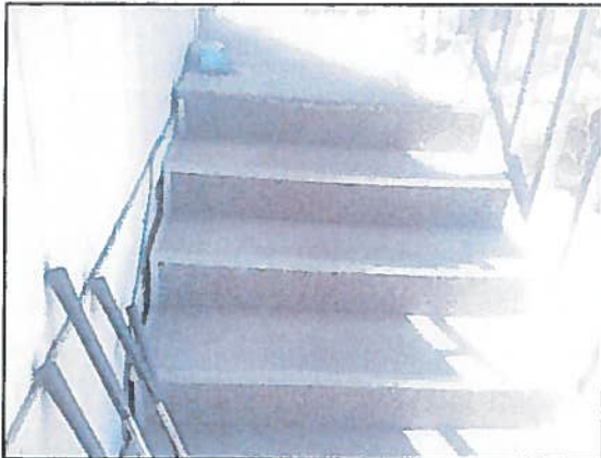
Photo 9 Fire Station 4 – Stairs to side door with damage and highly worn carpeting
