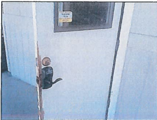
Photo 11 Fire Station 4 – Chipped and damaged wood door to garage
