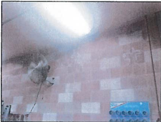
Photo 11 Maintenance Facility – Block wall efflorescence likely due to moisture infiltration
