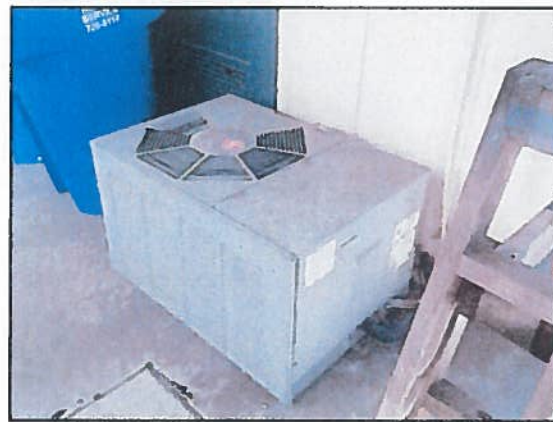
Photo 12 Fire Station 2 - Split system of 2001 manufacture
