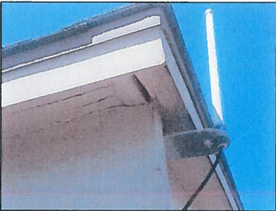
Photo 3 Fire Station 2 – Mild wood damage at soffit corner
