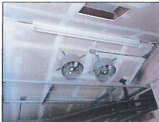
Photo 6 Communications Annex – Exhaust fans that would not start
