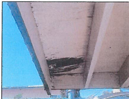
Photo 4 Communications Annex – Rotted and warped sheathing at roof corner
