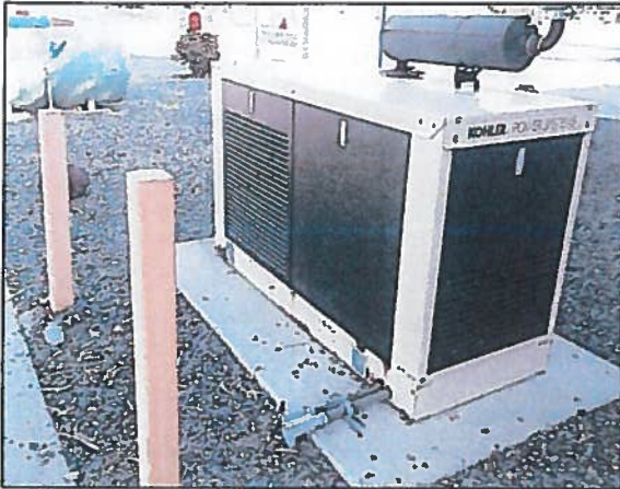
Photo 9 Fire Station 6 – Rust damage beginning
