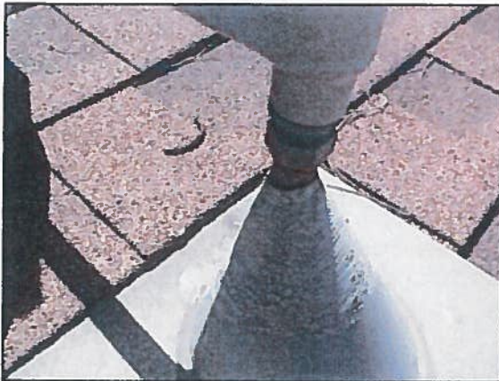
Photo 5 Fire Station 2 – Minor spot patching needed at roofing
