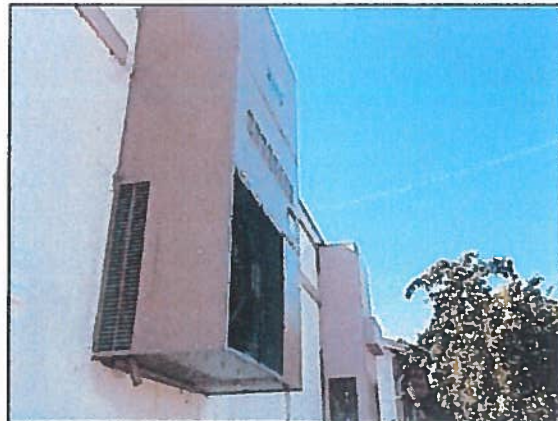
Photo 2 Rainbow Training Annex – Thru-wall package HVAC unit condensate drain lines need to be extended to prevent further water damage to wall
