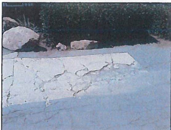
Photo 1 Roy Noon Meeting Hall – Heavy cracking, spalling and settlement at small section of front driveway
