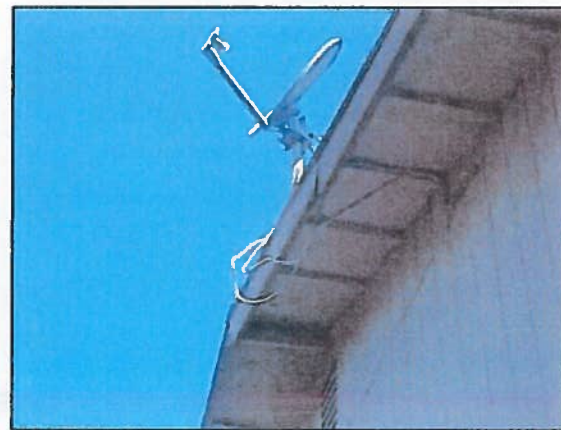
Photo 4 Fire Station 6 – Minor fascia board dislocation
