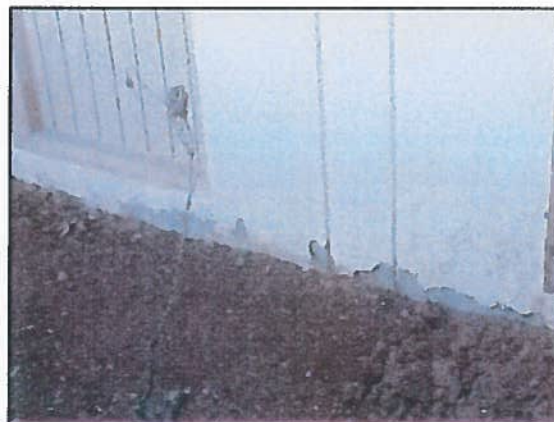
Photo 8 Fire Station 1 – Peeling paint along base of exterior wall
