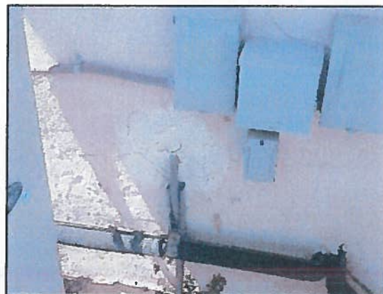
Photo 4 Communications Annex – Minor cracking within wall penetration seal
