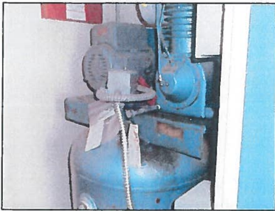
Photo 13 Fire Station 2 – Compressed air system shows little usage
