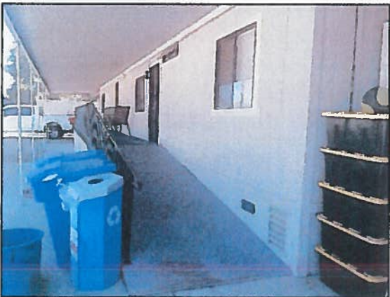
Photo 3 Fire Station 4 – Ramp for front door showing wearing and tear
