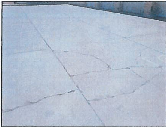
Photo 1 Storage Building – Moderate cracking throughout concrete driveway
