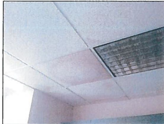
Photo 14 Fire Station 1 – Water-damage ceiling tile due to leaking
