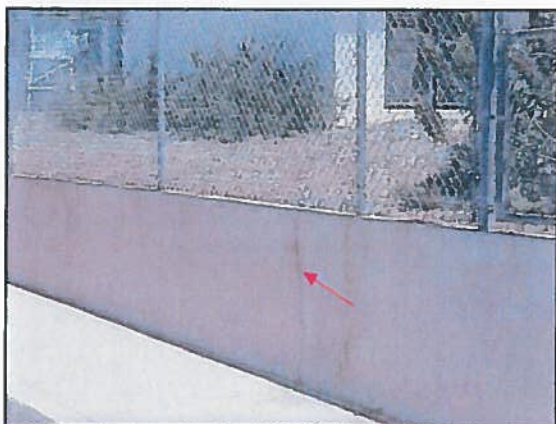
Photo 3 Fire Station 1 – Retaining wall cracks
