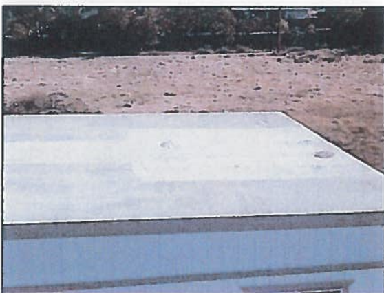
Photo 3 Rainbow Training Annex – Roof in poor condition with visible patches and evidence of ponding
