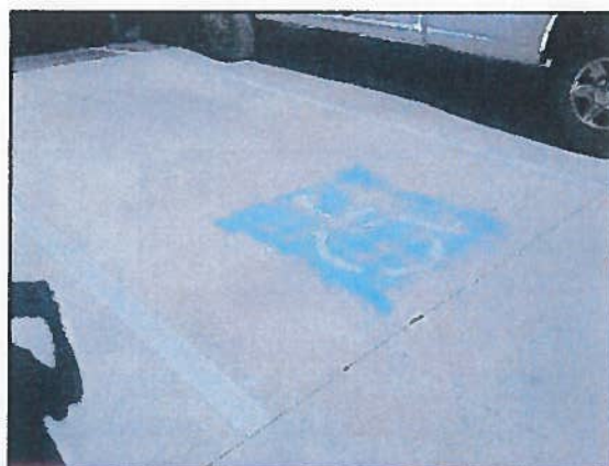
Photo 4 Fire Station 1 – Faded parking striping/marking
