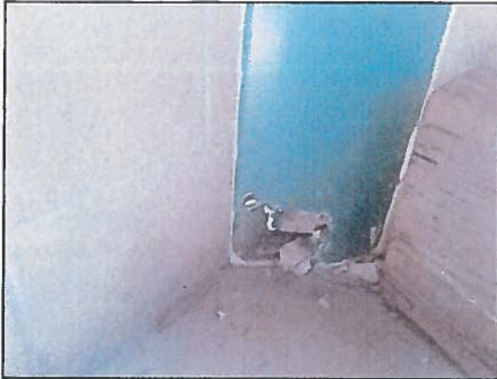
Photo 5 Maintenance Facility – Damage to exterior staircase column shell
