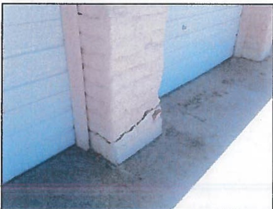
Photo 3 Storage Building – Large crack through section of adobe block between overhead doors
