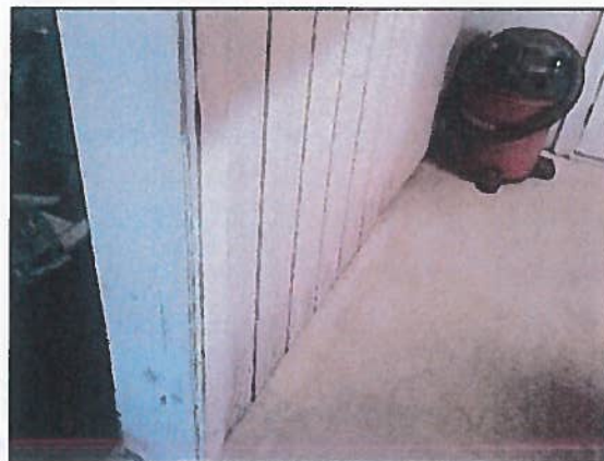
Photo 12 Fire Station 4 – Some visible wear on siding within garage, apparently due to reported roof leak
