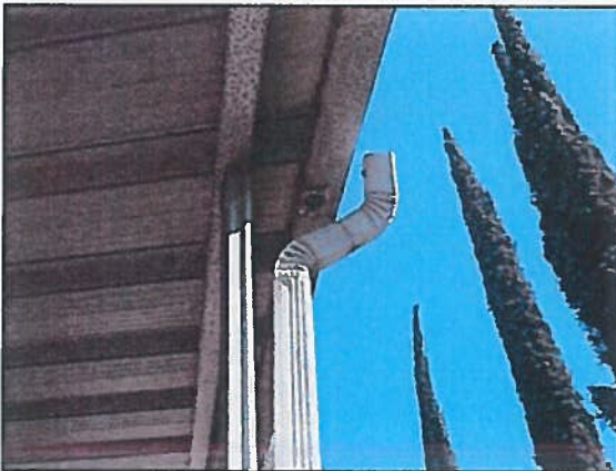
Photo 15 Fire Station 4 – Damage/displacement of overhang gutter on west side
