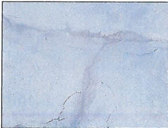
Photo 3 Fire Station 3 – Crack sealant in asphalt parking area has failed in some areas and new, mild cracks seem to have formed.
