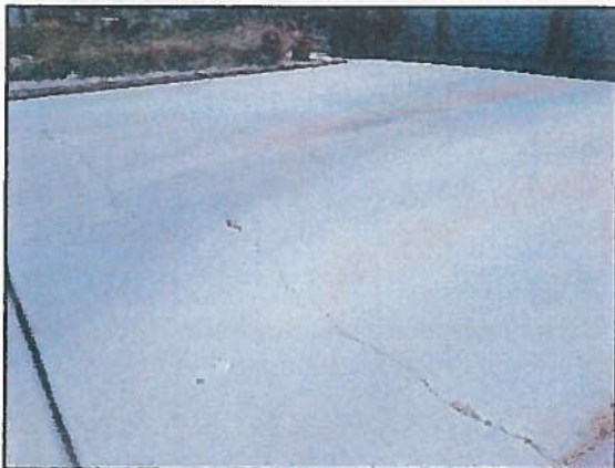
Photo 1 Fire Station 1 – Cracking at front driveway
