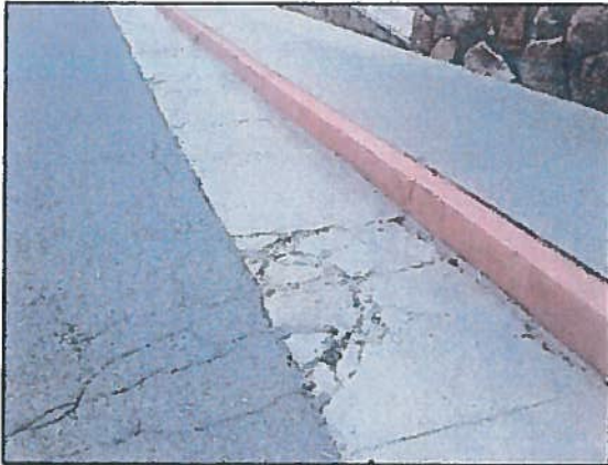
Photo 1 Communications Annex – Concrete along curb with spalls and cracks
