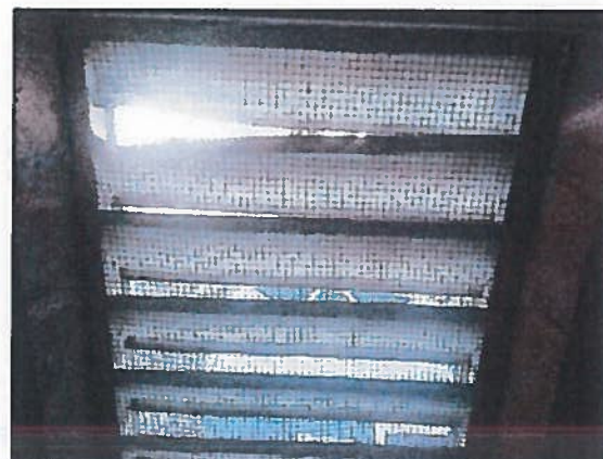
Photo 8 Fire Station 2 - Penetration in equipment room vent
