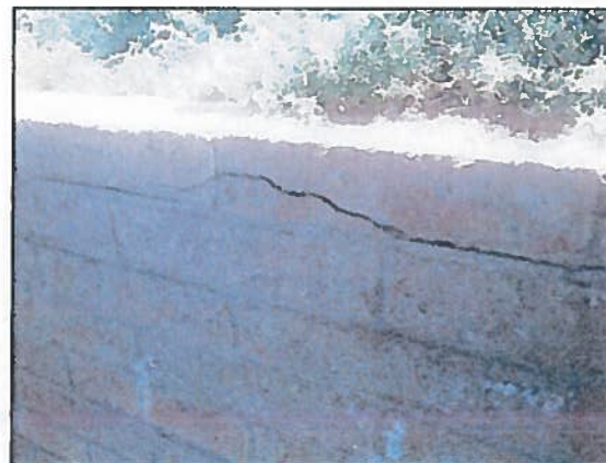
Photo 4 Fire Station 3 – Crack at top of back retaining wall
