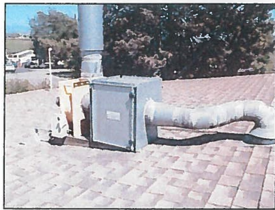
Photo 14 Fire Station 2 - Exhaust/Tail pipe system exposed ducting sealant failing
