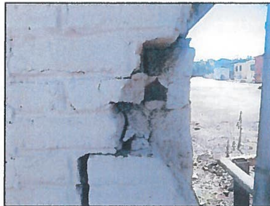
Photo 2 Storage Building – Damaged southwest wall corner due to either settle or vehicle impact
