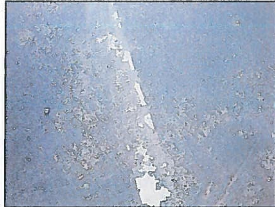
Photo 6 Fire Station 3 – Faded and flaking parking area asphalt seal coat and striping
