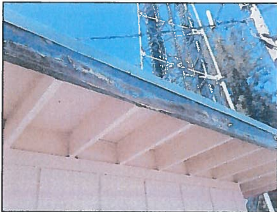
Photo 3 Communications Annex – Rotted fascia board
