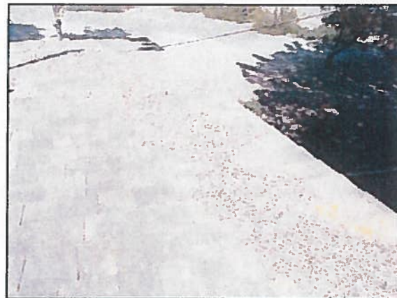
Photo 6 Fire Station 2 – Debris buildup on roof
