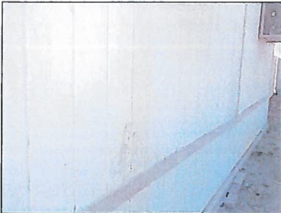
Photo 1 Rainbow Training Annex – Minor water damage to siding due to package unit condensate dripping
