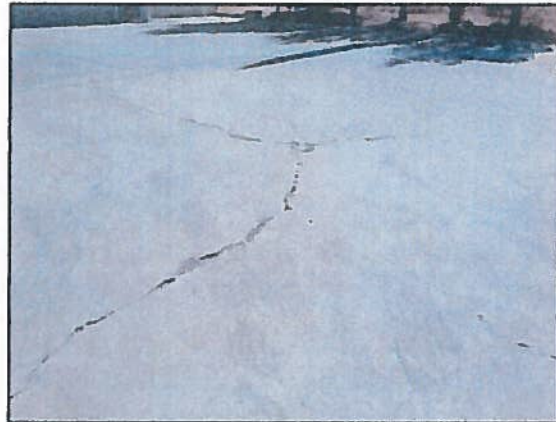
Photo 2 Fire Station 4 – Moderate severity cracks and spalls throughout a large percentage of driveway
