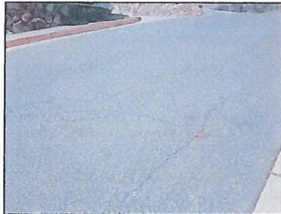
Photo 2 Communications Annex – Moderate cracking in asphalt driveway
