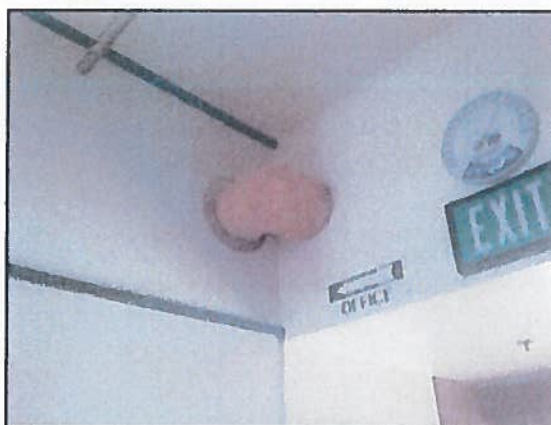
Photo 14 Maintenance Facility – Duct join in need of cover
