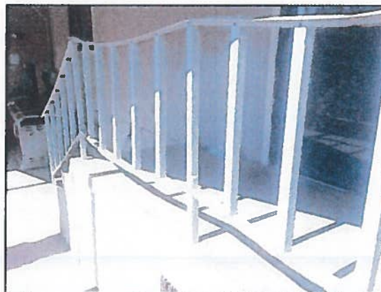
Photo 8 Fire Station 4 – Damaged side door landing railing
