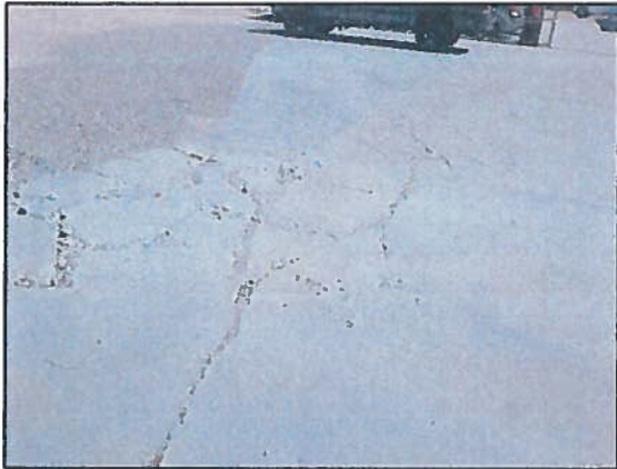
Photo 1 Fire Station 4 – Cracks and spalls along east edge of concrete driveway
