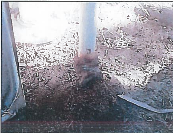
Photo 3 Fire Station 6 – Rusted and blocked end of fire sprinkler drain
