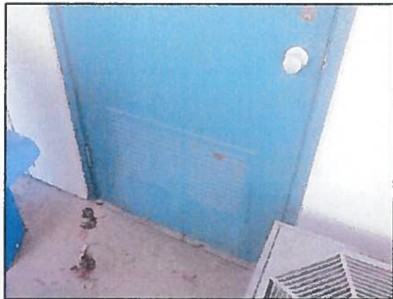
Photo 4 Fire Station 2 - Mild rusting at exterior door louver
