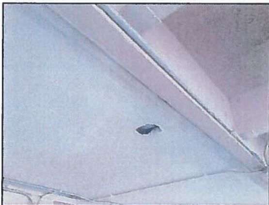
Photo 7 Fire Station 1 – Hole in south side soffit
