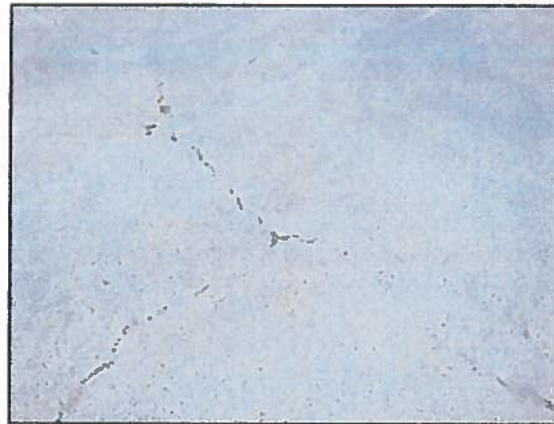
Photo 2 Fire Station 3 – Cracks in back driveway concrete
