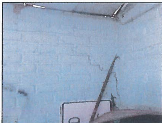
Photo 4 Storage Building – View of cracking on interior side of damaged wall corner
