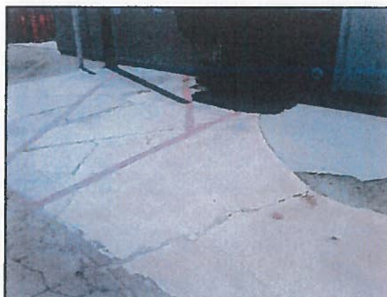
Photo 2 Roy Noon Meeting Hall – Cracks throughout front driveway
