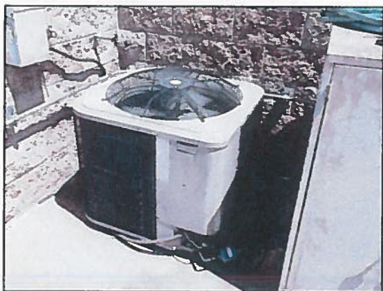
Photo 15 Maintenance Facility – The refrigeration tubing insulation outdoors needs to be replaced and UV protected
