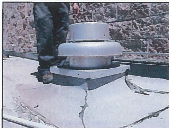
Photo 16 Maintenance Facility - The low roof section acorn exhaust fan failed a run test. This ventilates the Electric Room and Air Compressor Room
