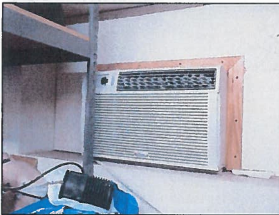
Photo 7 Storage Building – Unit is not in service at this time. Life Cycle estimated at 7-10 years
