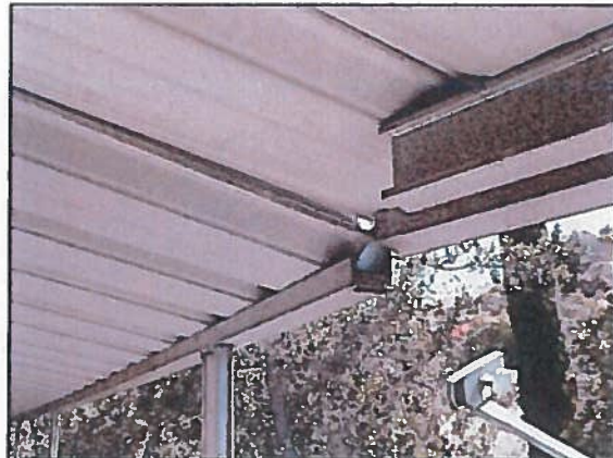
Photo 14 Fire Station 4 – Questionable overhang transition on west side where possible damage/displacement has occurred
