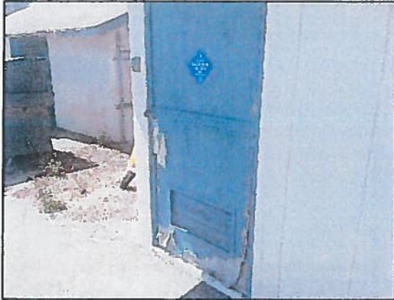
Photo 5 Communications Annex – Front door exhibiting heavy degradation.
