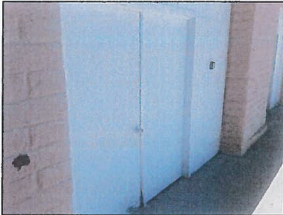
Photo 5 Storage Building – Some damage to base of exterior double door
